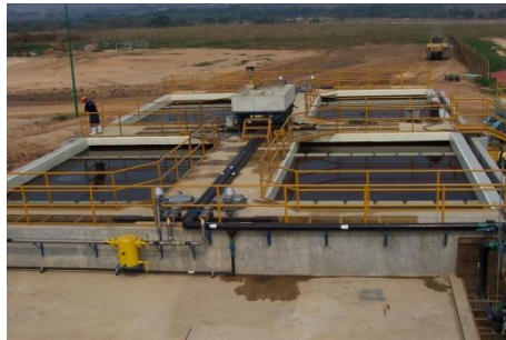
UASB anaerobic reactors
