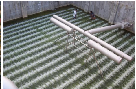
Sequencing Batch Reactor (SBR)
